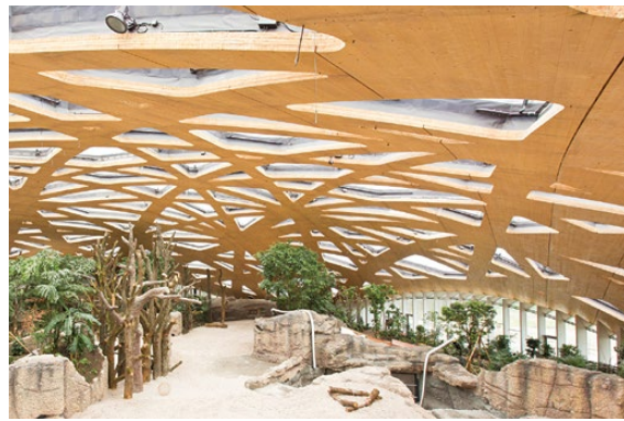
The wood construction at the new elephant house at the Zurich Zoo has been built using Loctite Purbond adhesive, which was transported in Fluid-Bags.
